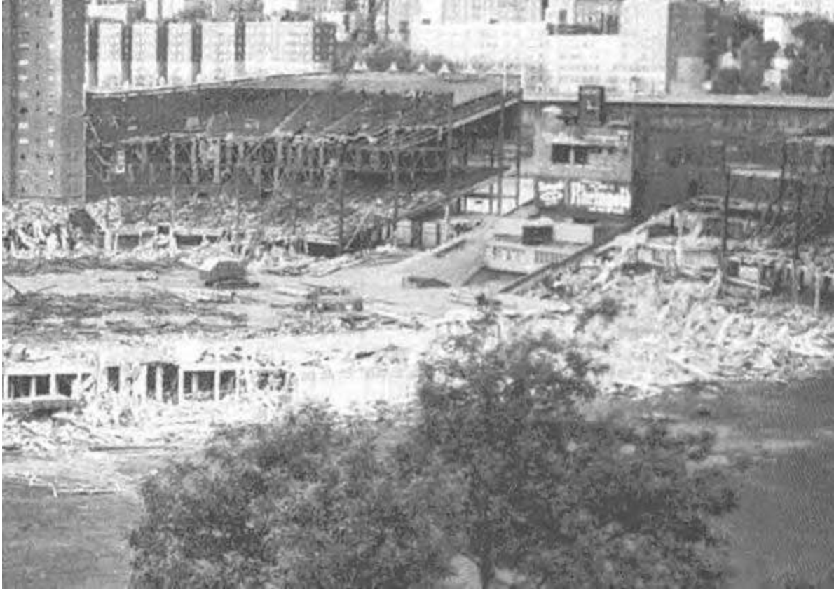
The Polo Grounds under demolition – a tragic sight for fans of many teams.
