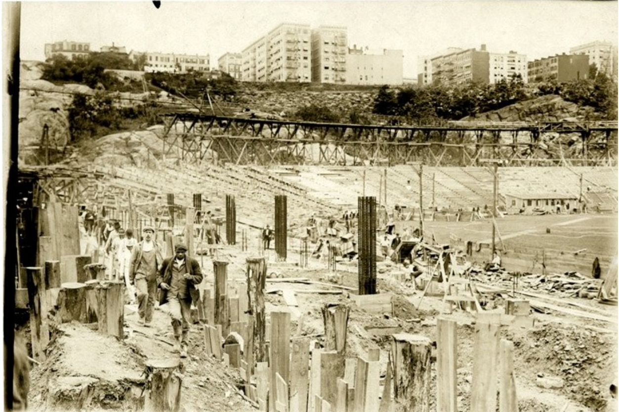
Another view of the demolition of the Polo Grounds. The Brush Staircase should be visible above the disintegrating stands.
