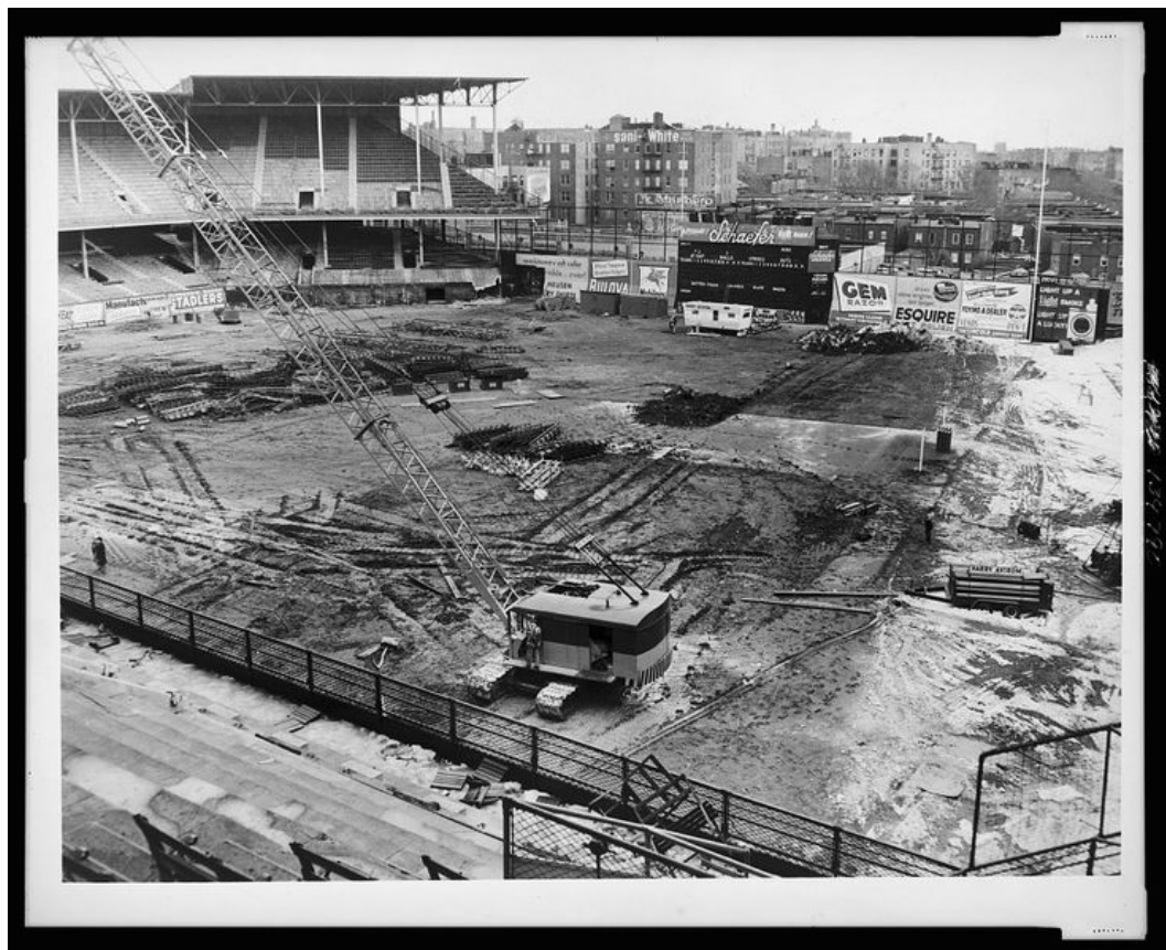
The most horrific sight for all Brooklyn Dodger fans: the stadium being demolished in 1960.
